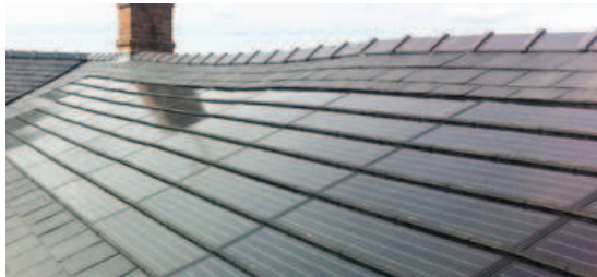
Solar PV system (C21e slate)
